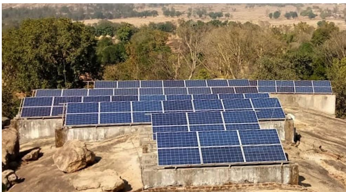
Community mini-grid installed in Sahtioli village Source: Mlinda, 2019
