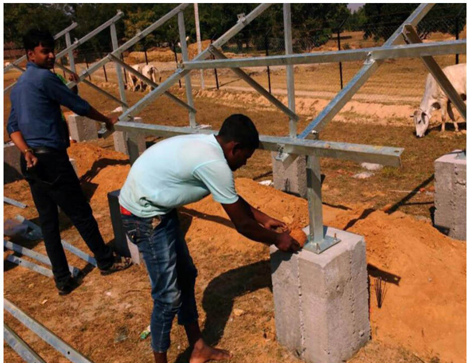
Local workers installing the framing for photovoltaic (PV) solar panels Source: Mlinda, 2019
