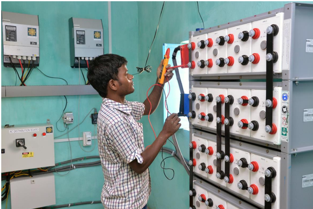
Mini-grid plant operator checks battery charge in mini-grid power house Source: Mlinda, 2019
