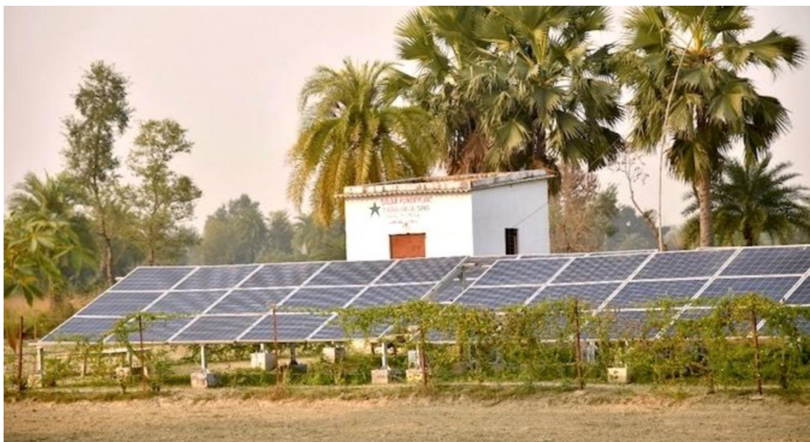
Solar mini-grid in India Source: Smart Power India, 2018
